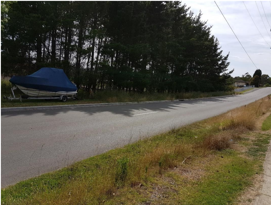
Image 2: Quarry Road has a road sag east of the southern site boundary
