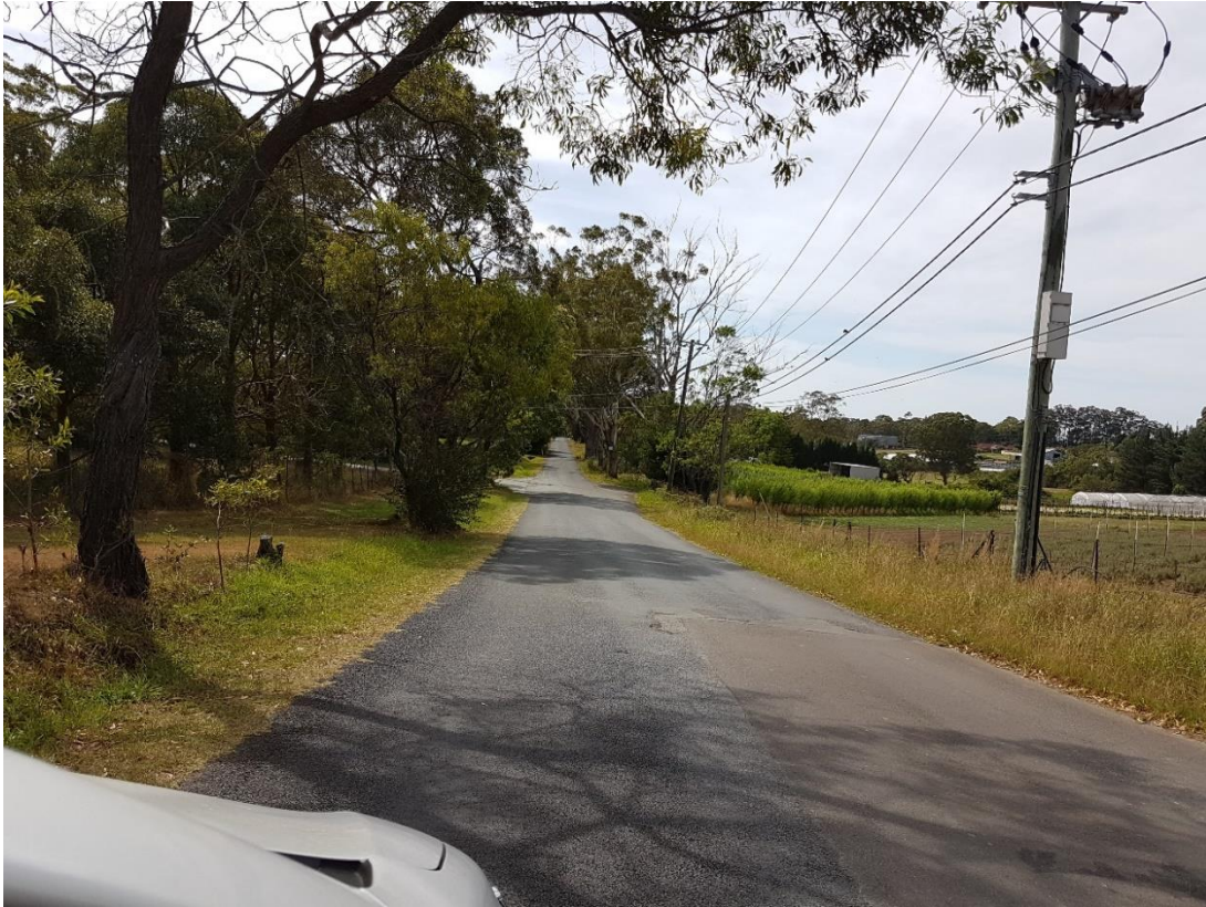
Image 5: Vineys Road has a road sag near the cross intersection at Vineys Lane.
